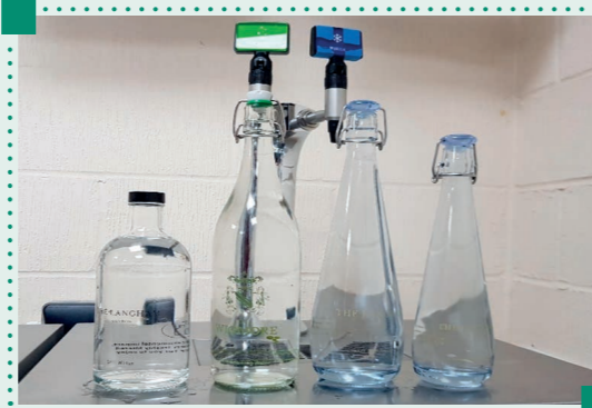
Water bottling system at The Langham, London
