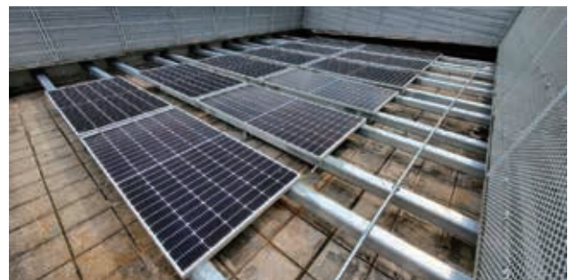
Solar Panels at Rooftop
