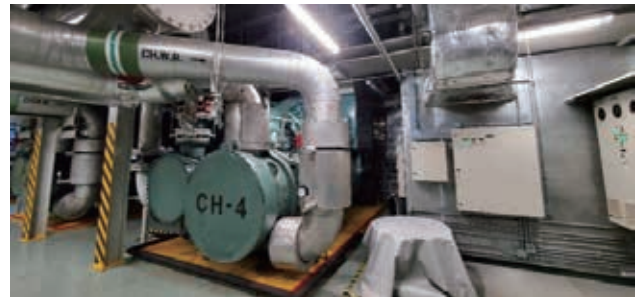
Smart lighting at Chiller Plant
