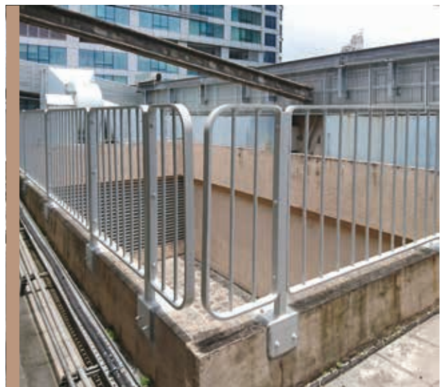
Protective Barrier on the Roof
